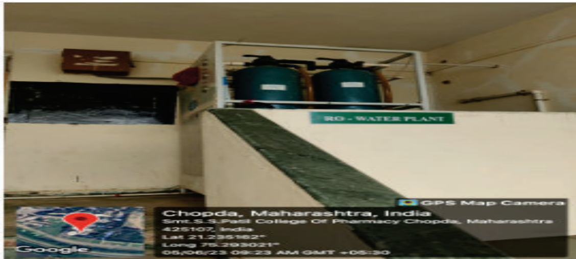
Water purification plant
