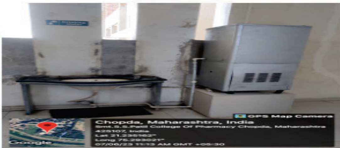
Drinking water Plant
