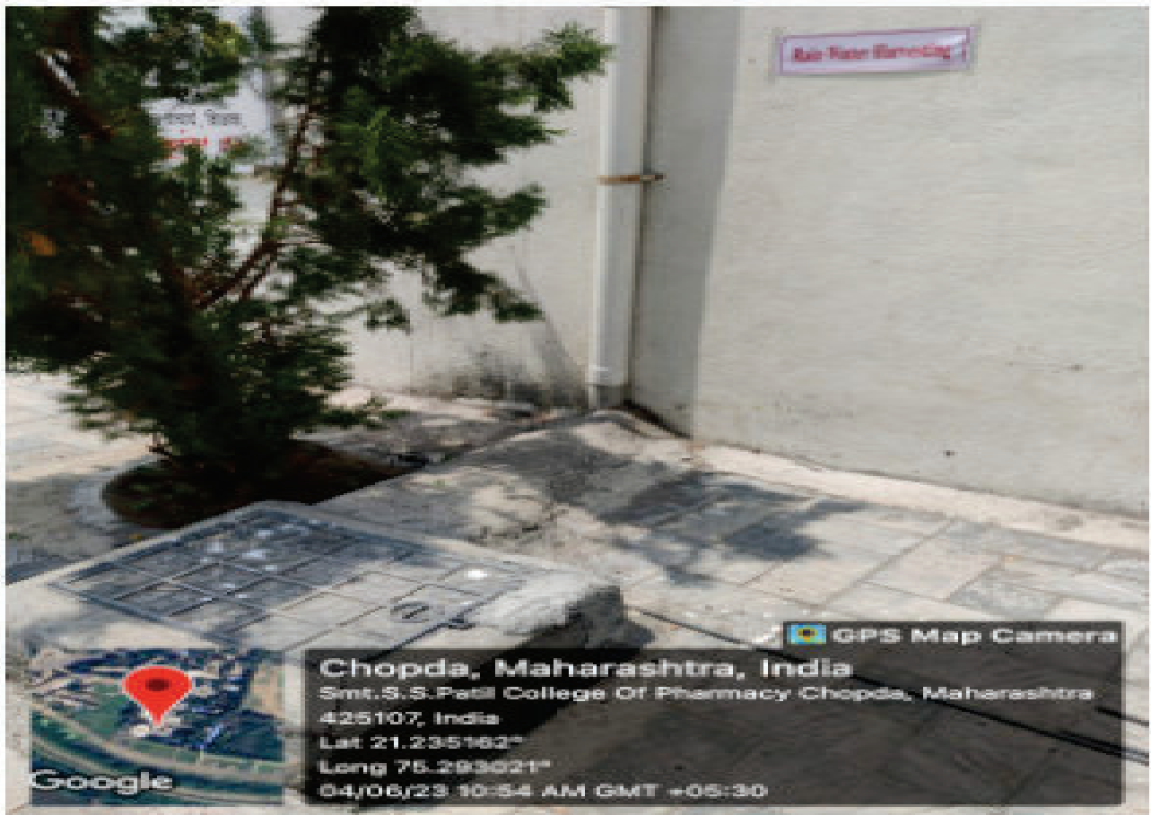
Rain Water Harvesting
